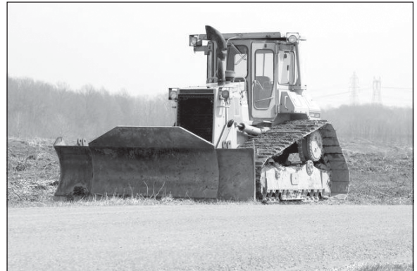
Fine dust particles from construction sites can trigger chronic bronchitis, emphysema, and heart disease. CEQA has been used to ensure that developers employ proper mitigation strategies, minimizing the health risks faced by workers and nearby residents.
